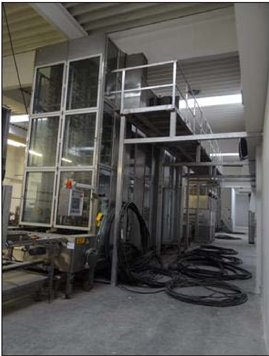
Picture 4. Automatic storage facility with top conveyance using an electric pusher
